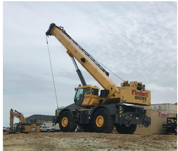
We have one of the many cranes that will be on site throughout the project. This crane will be used to help with footings that are starting next week!
