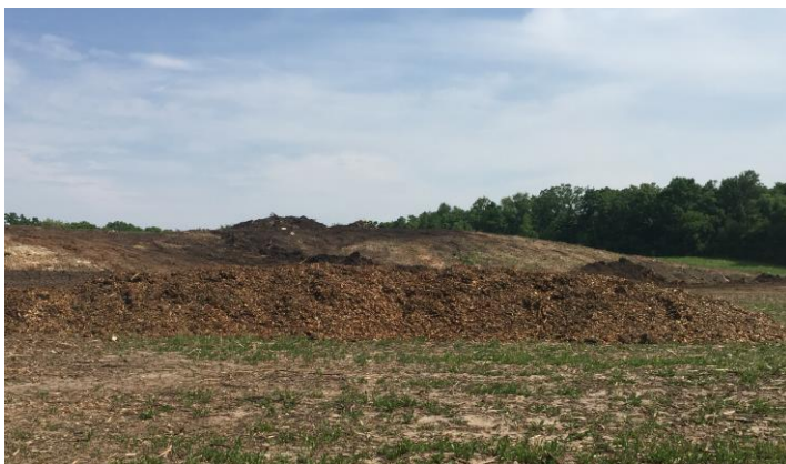
The future baseball diamond from the ground, this hill will soon be graded to match surrounding elevations
