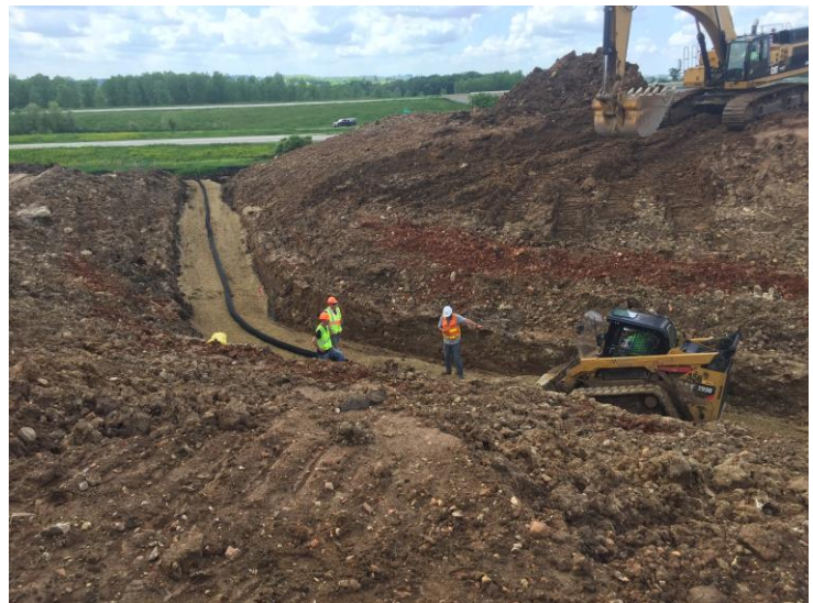
Installation of the French drain on the west side of the site
