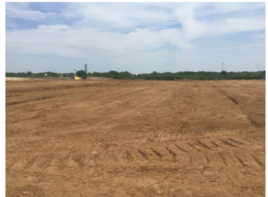
What used to be a hilly cornfield is now level and near ready for foundations
